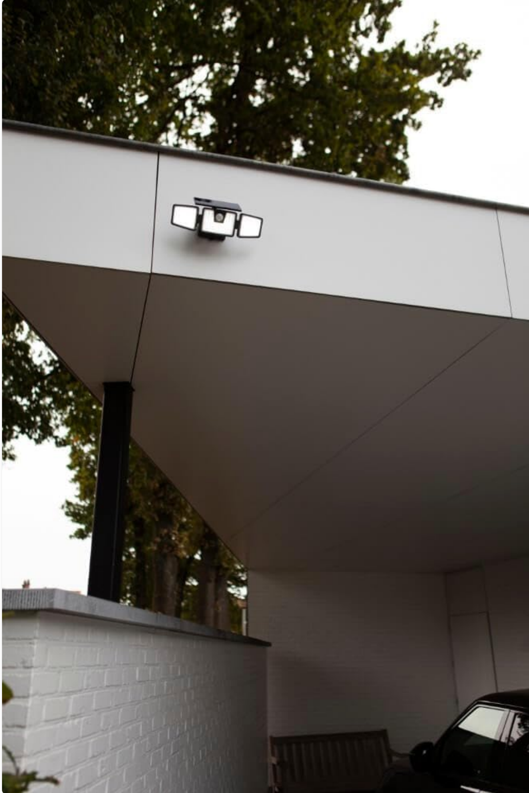
Image: The Lutec Briti 3 Solar Wall Lamp mounted on an exterior wall, demonstrating its discreet integration into a modern architectural setting. The solar panel is visible at the top, angled to capture sunlight.
