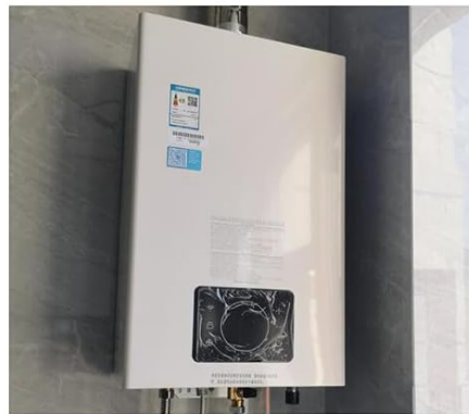
GAS WATER HEATER
