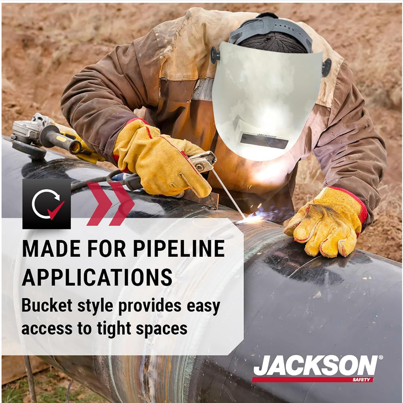
Figure 2.2: A welder utilizing the Jackson Safety PL280 helmet for pipeline applications, demonstrating its compact design for tight spaces.
