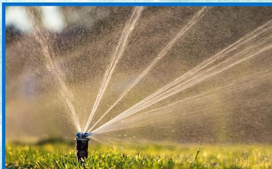
Garden Irrigation System
