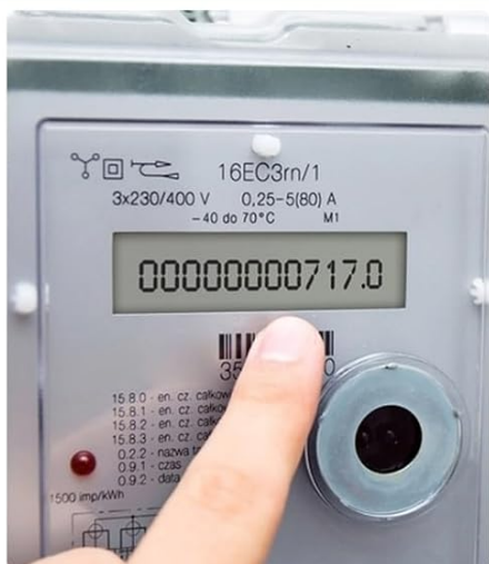
Electric power metering system
