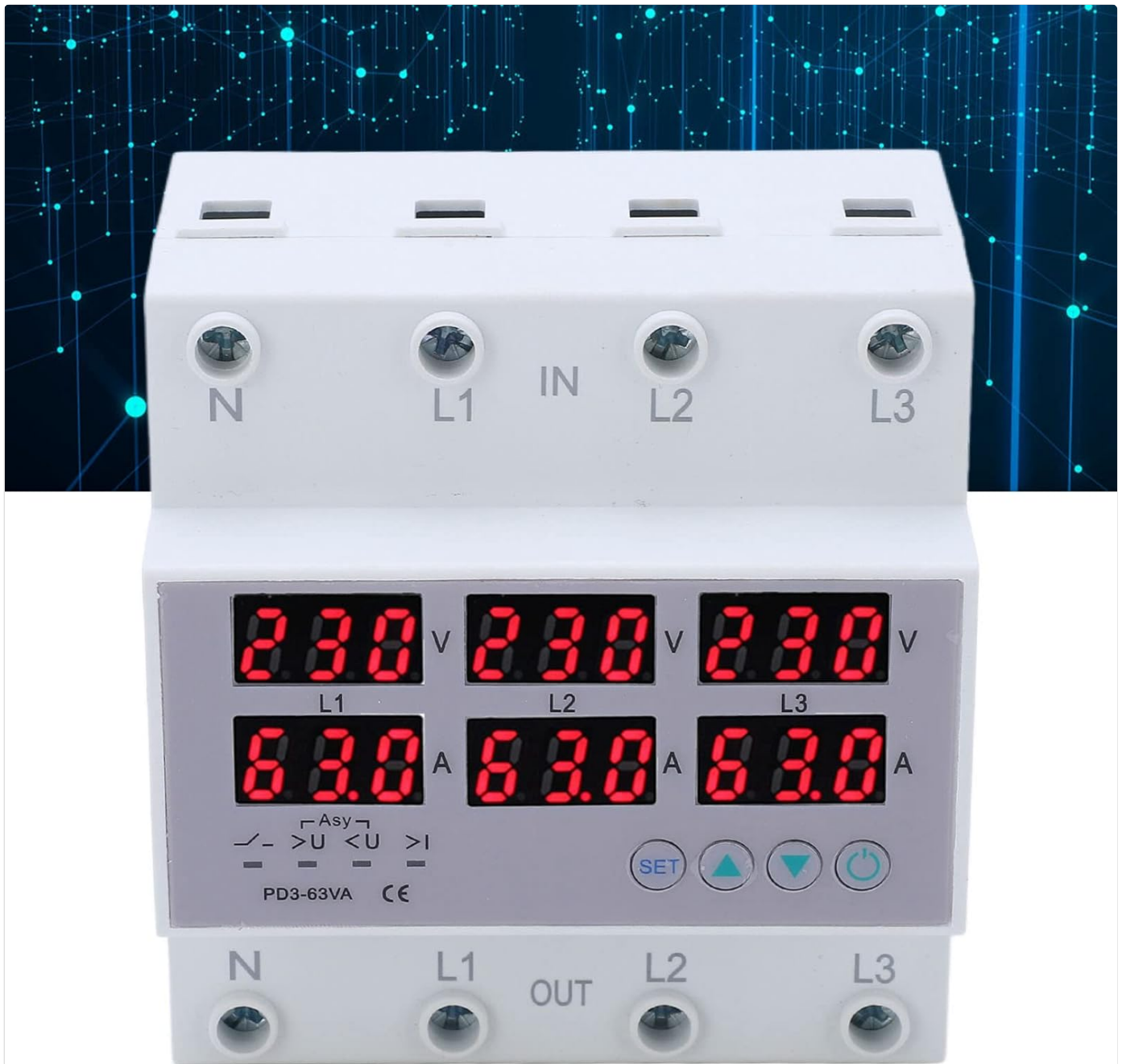
Figure 4: Digital display showing real-time voltage and current values for L1, L2, and L3.
