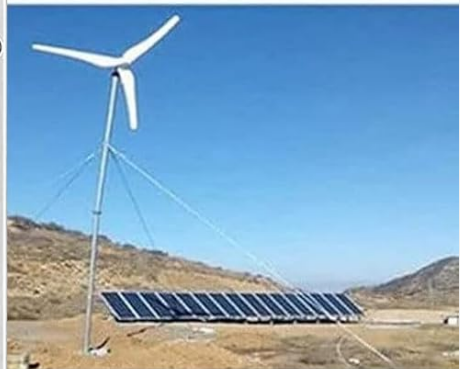
High-altitude mountainous area Photovoltaic Power Generation
