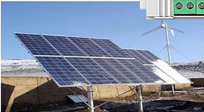
roof home Wind-solar hybrid power generation
