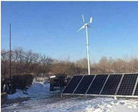
Wind-solar hybrid power generation in poor climate environment
