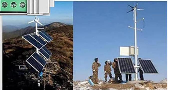
outdoor monitoring Wind-solar hybrid power generation
