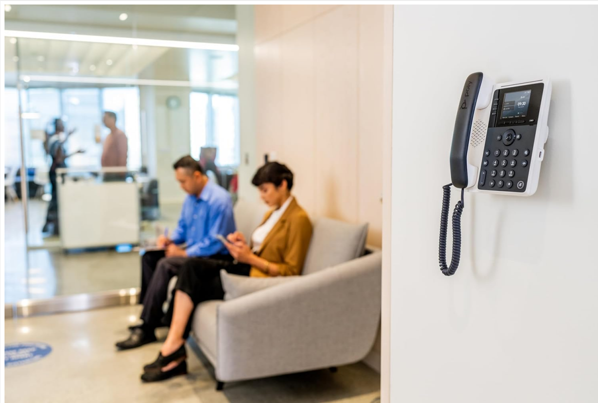
Figure 3: Poly Edge E100 IP Phone installed on a wall.
