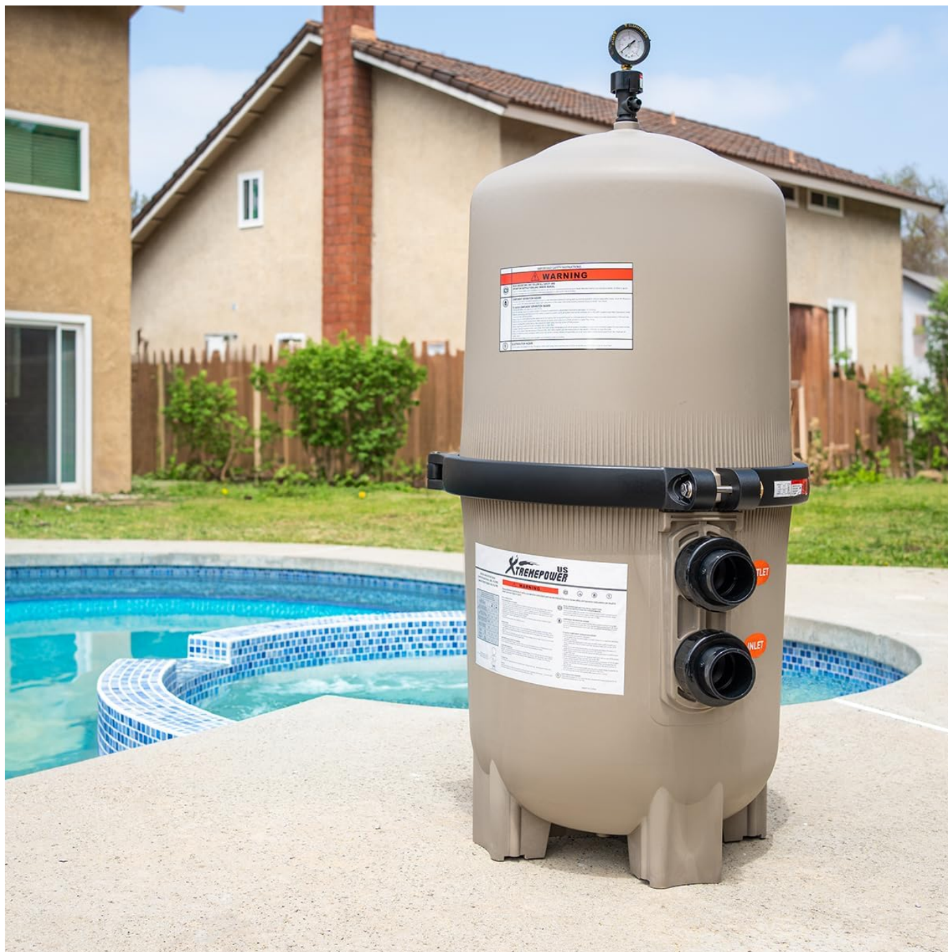
Image 4.1: Example of a DE pool filter installed adjacent to a swimming pool.
