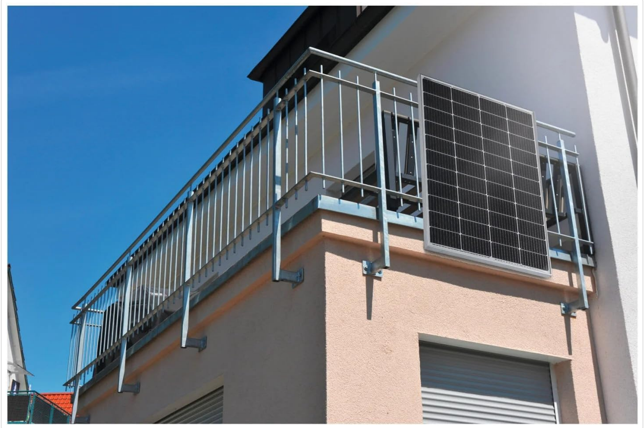
Image: A solar panel mounted on a balcony, showing its integration with the building structure.
