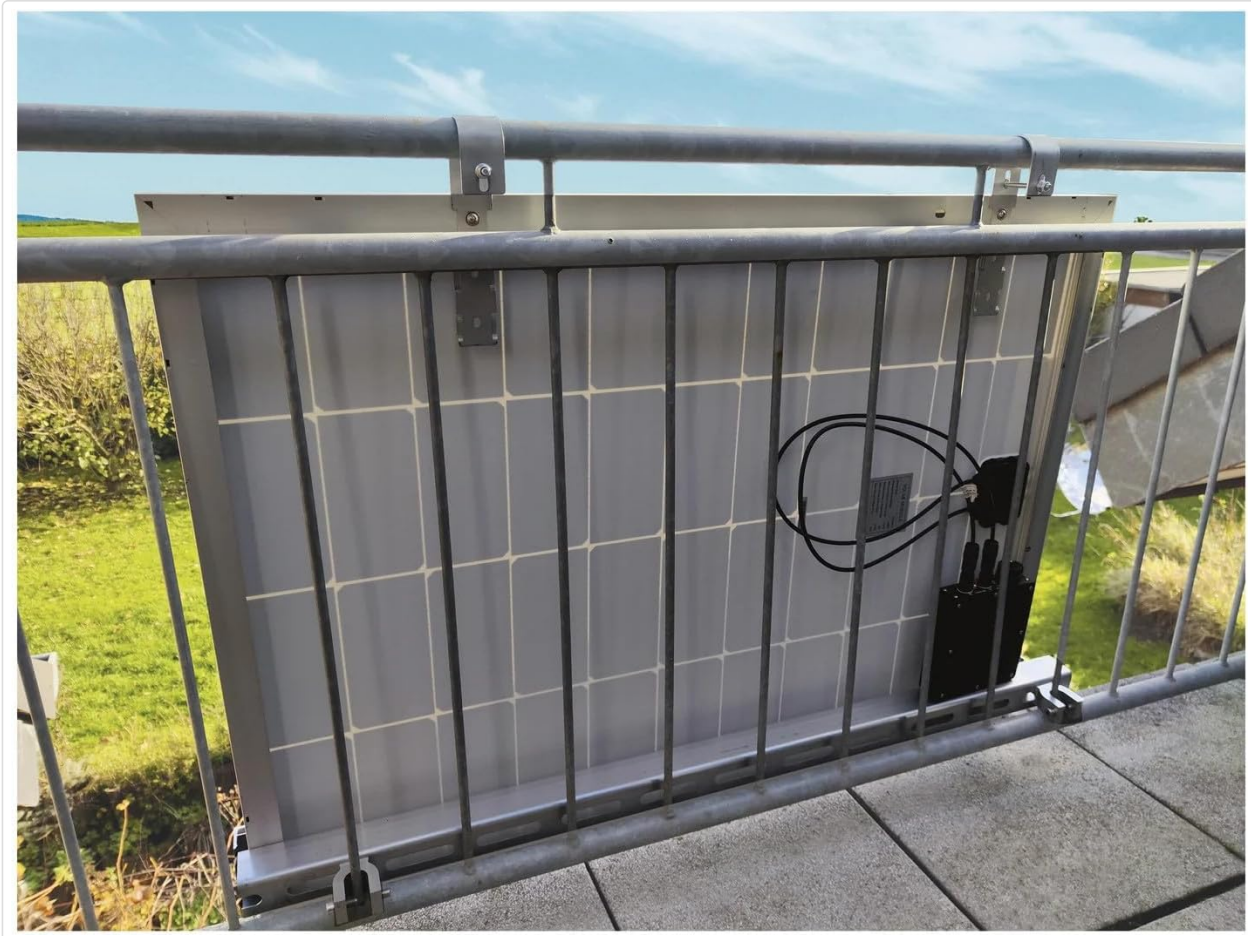
Image: Rear view of the solar panel with the micro inverter and wiring connected, as seen from the balcony.
