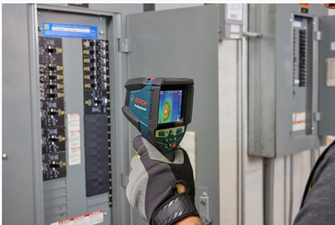
Figure 5.1: Using the thermal camera to inspect an electrical panel for hot spots.
