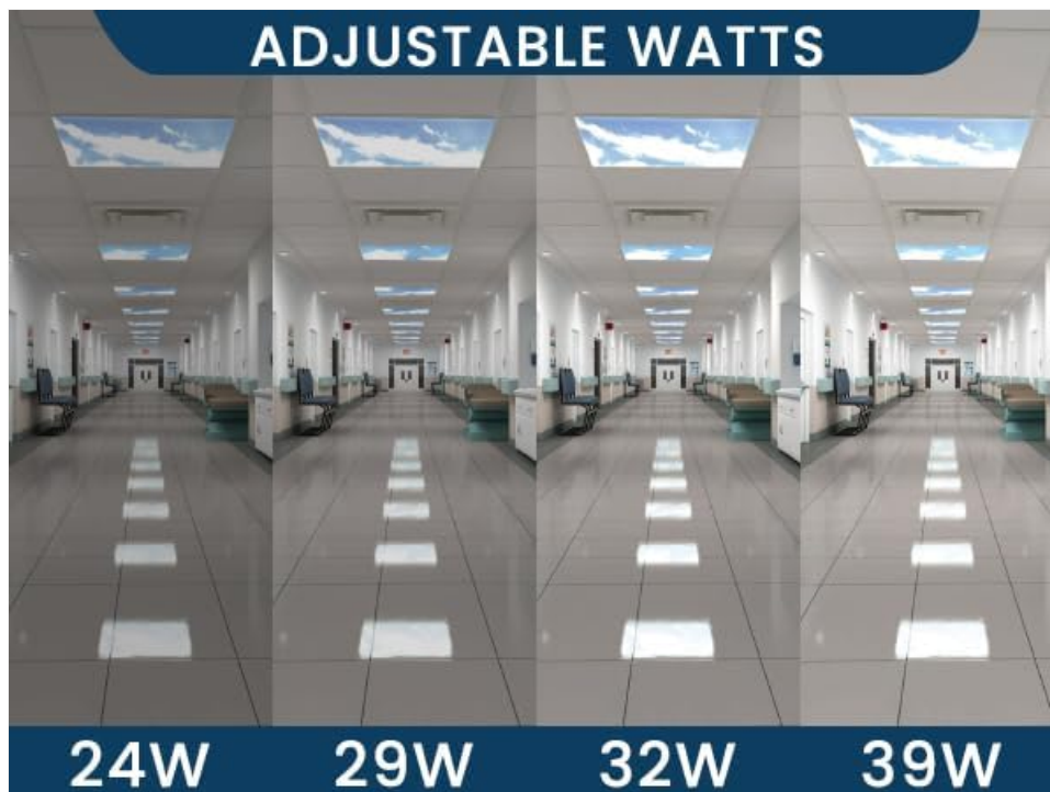
Figure 2: Adjustable Wattage settings (24W, 29W, 32W, 39W) for the LED panel light. This image illustrates how the light output changes with different wattage selections in a hallway setting, allowing users to choose their preferred brightness and energy consumption.
