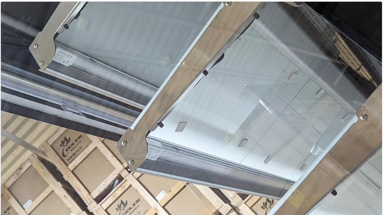
Figure 6: Internal LED lighting.
