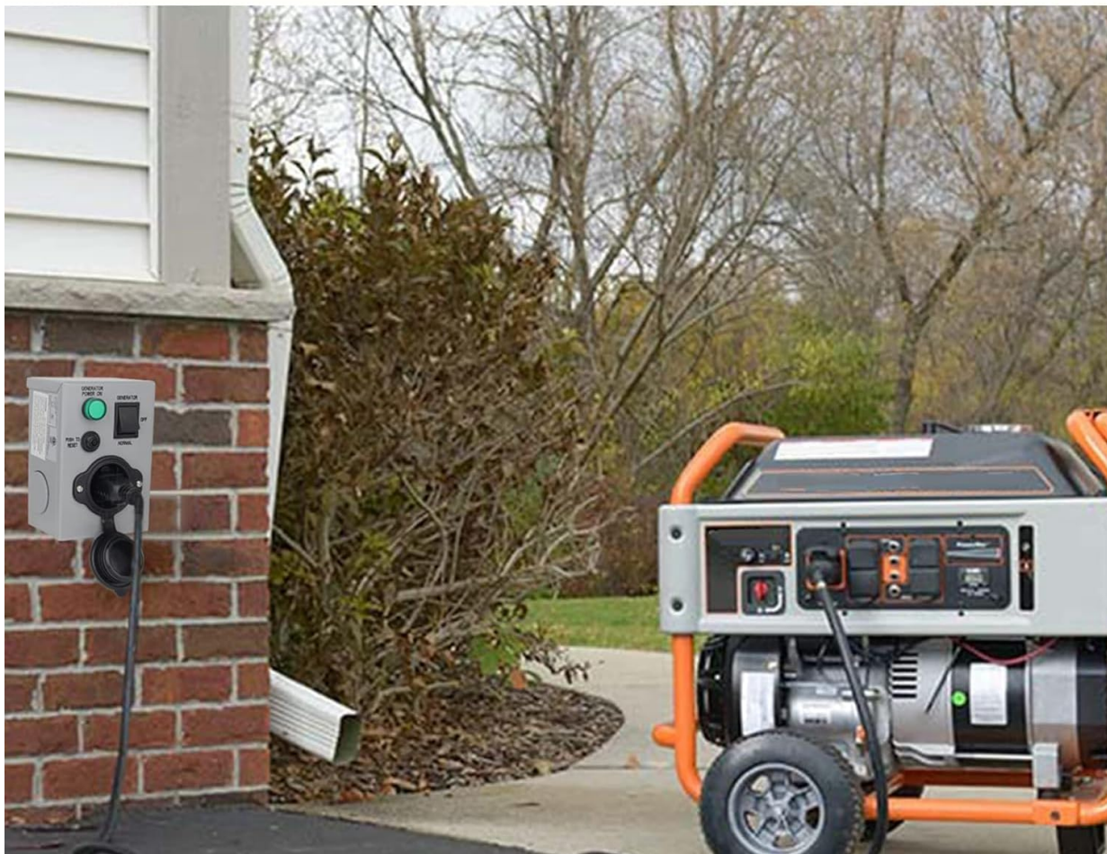
Figure 5: Outdoor Setup - Demonstrates the transfer switch installed on an exterior wall, connected to a portable generator.
