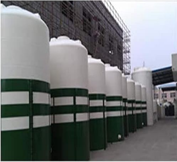
Intelligent Water Supply for Water Tower and Tank
