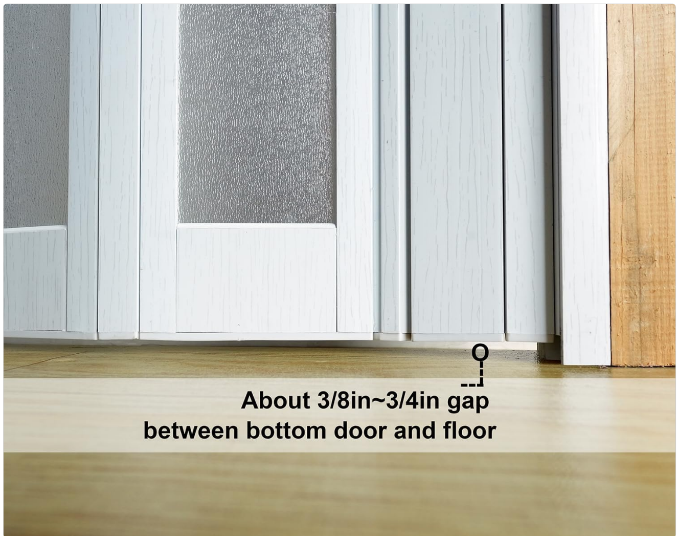
Figure 3.2: Bottom Door to Floor Gap. This image provides a detailed view of the recommended clearance between the bottom of the door and the floor, which is approximately 3/8 to 3/4 inches.
