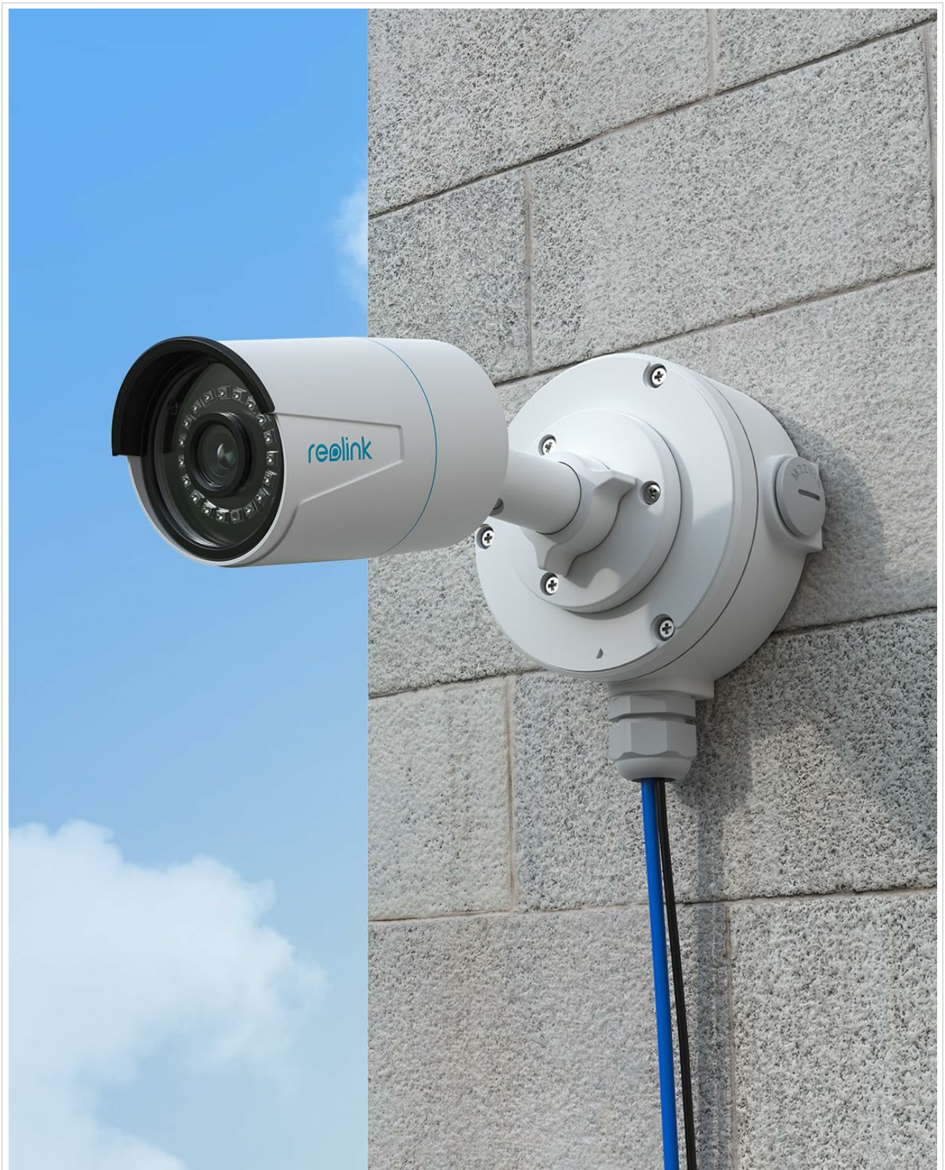
Figure 4: Installed REOLINK Junction Box with Camera
