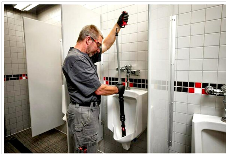
Figure 3: Example of using the M12 TRAPSNAKE™ Driver for drain clearing.
