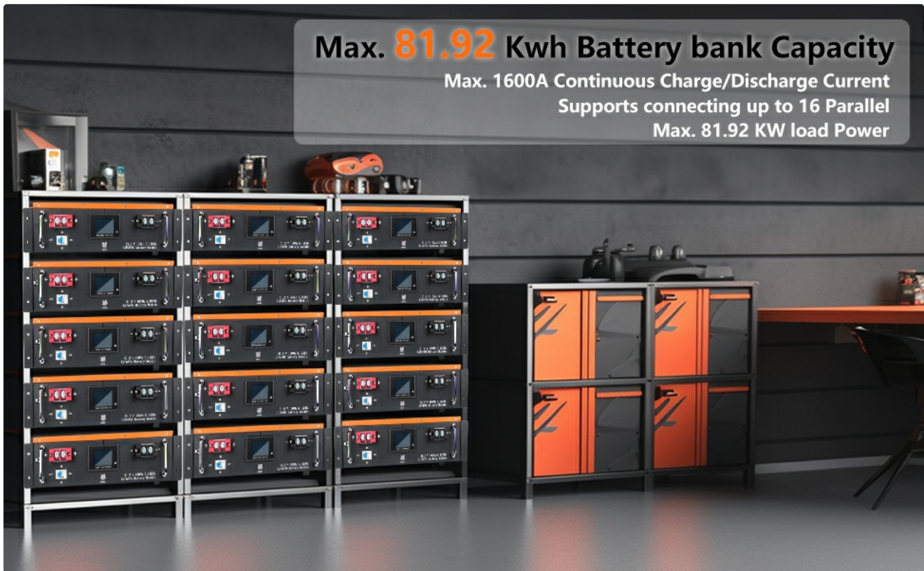
Figure 6: A setup showing multiple Cloudeenergy batteries installed in a rack, demonstrating scalability up to 16 units for increased capacity.
