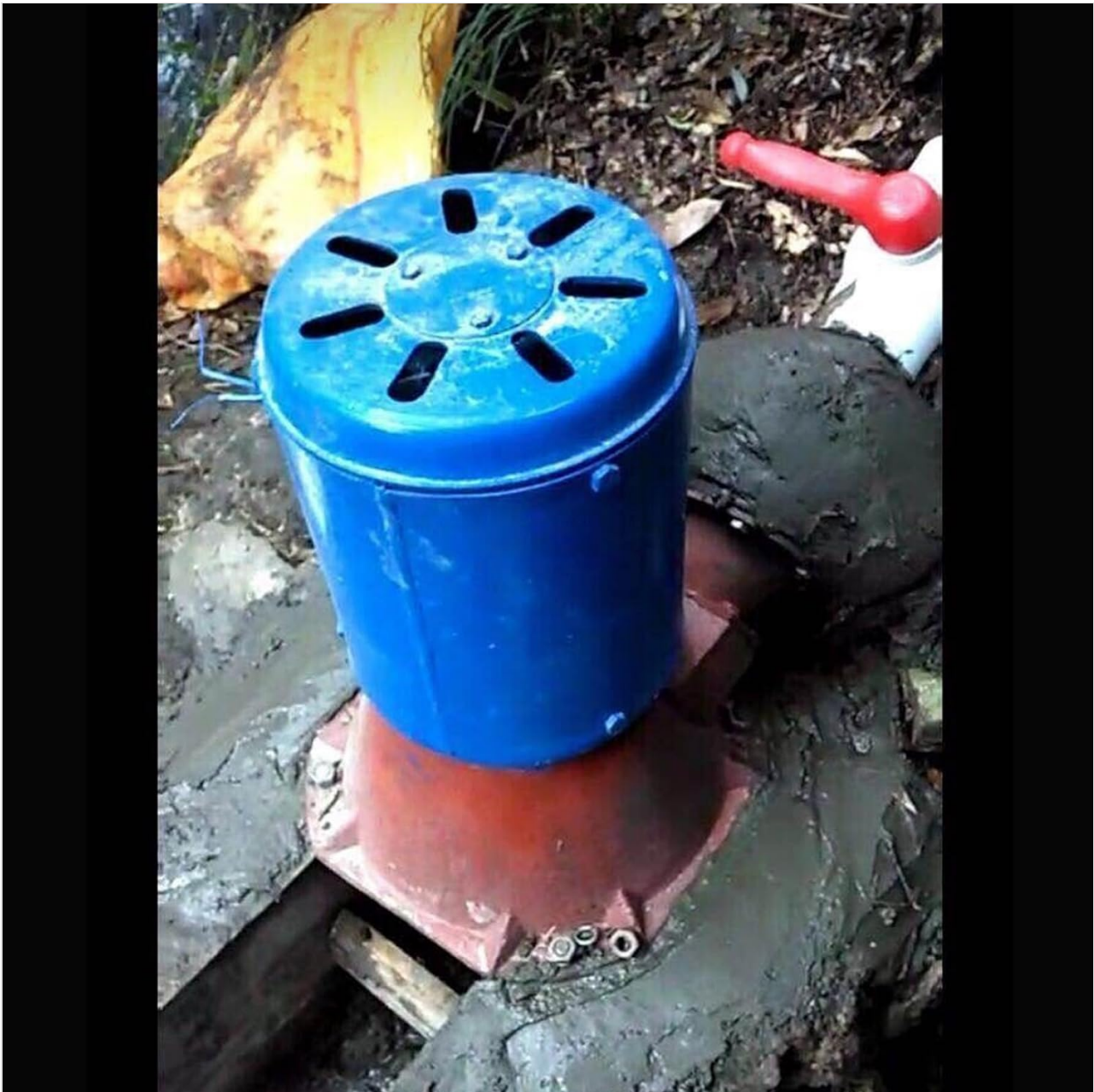
Figure 4.2.3: An OLONETO hydroelectric generator installed within a concrete water channel, demonstrating a typical setup with a red control valve.
