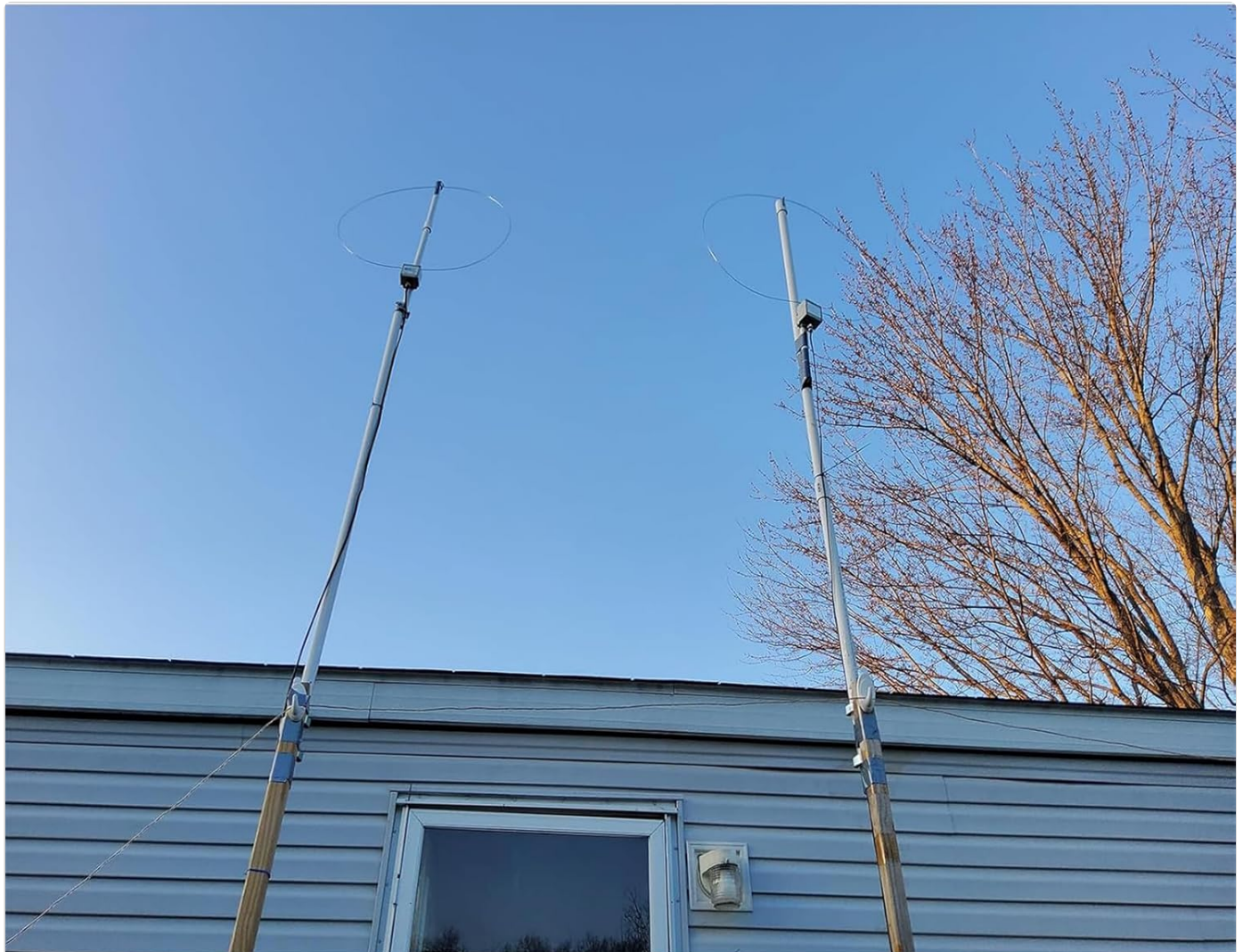
Figure 7: Example of K-480WLA antennas installed outdoors.
