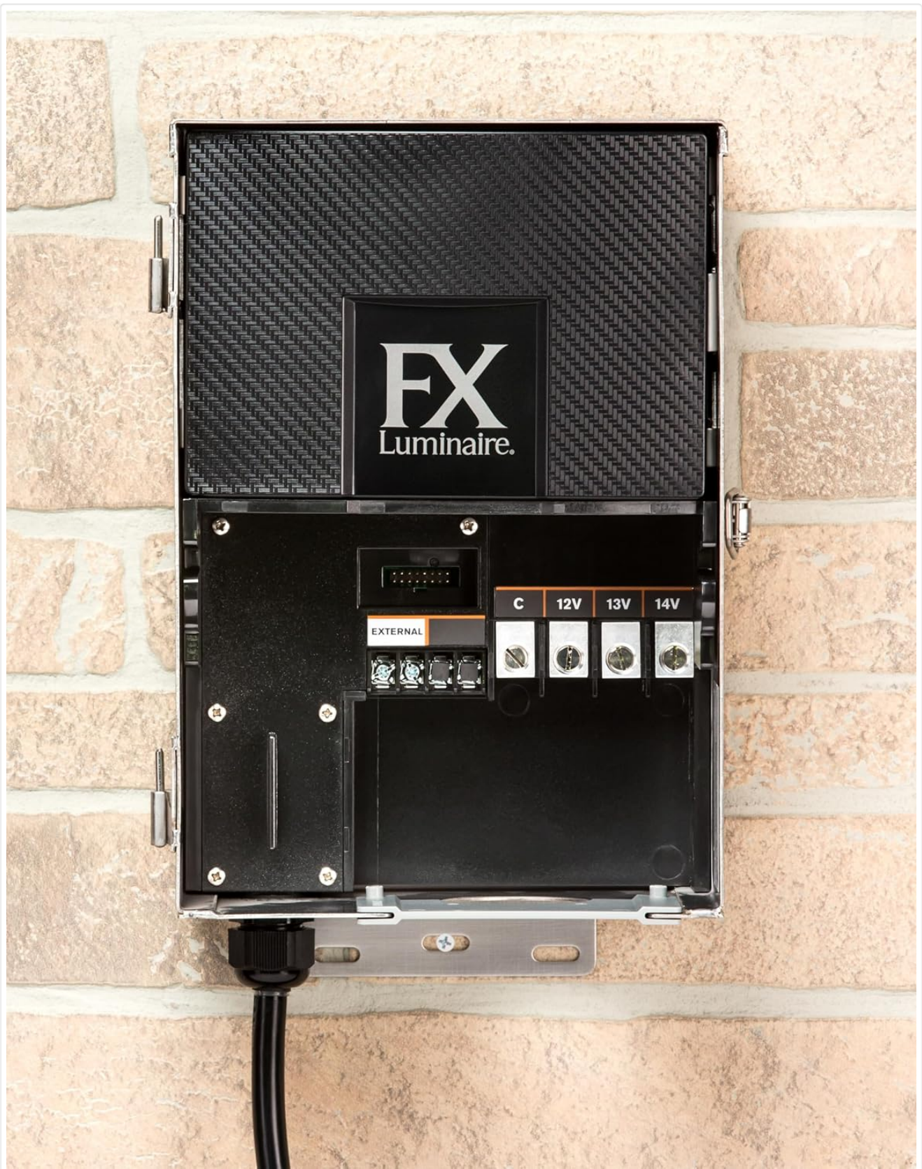
Figure 2: Internal view of the transformer, highlighting the low-voltage output terminals and the external input connection.
