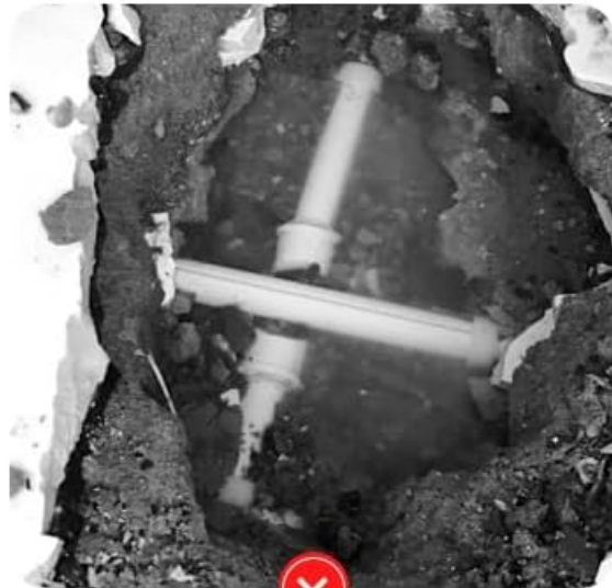
Leaking PVC water pipes
