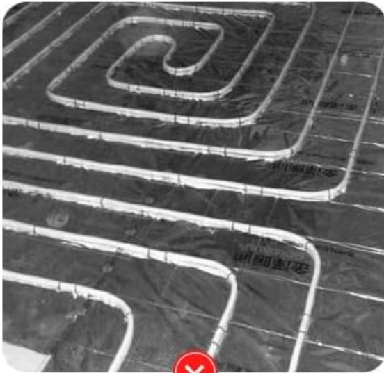
Leaking underfloor heating pipes
