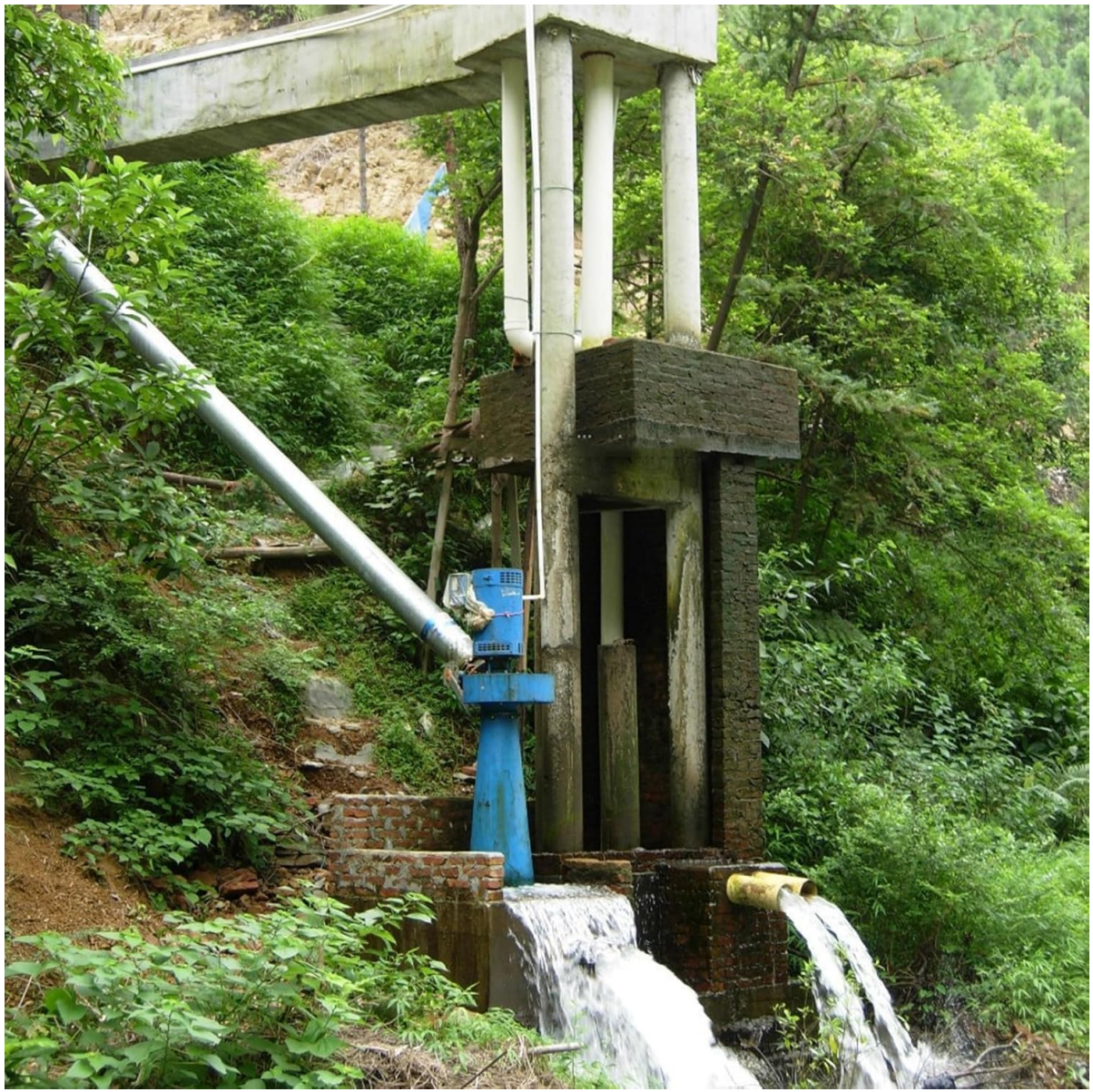
Figure 4.1: Example of a hydroelectric generator installation in a natural stream environment, showing the water intake pipe and generator unit.
