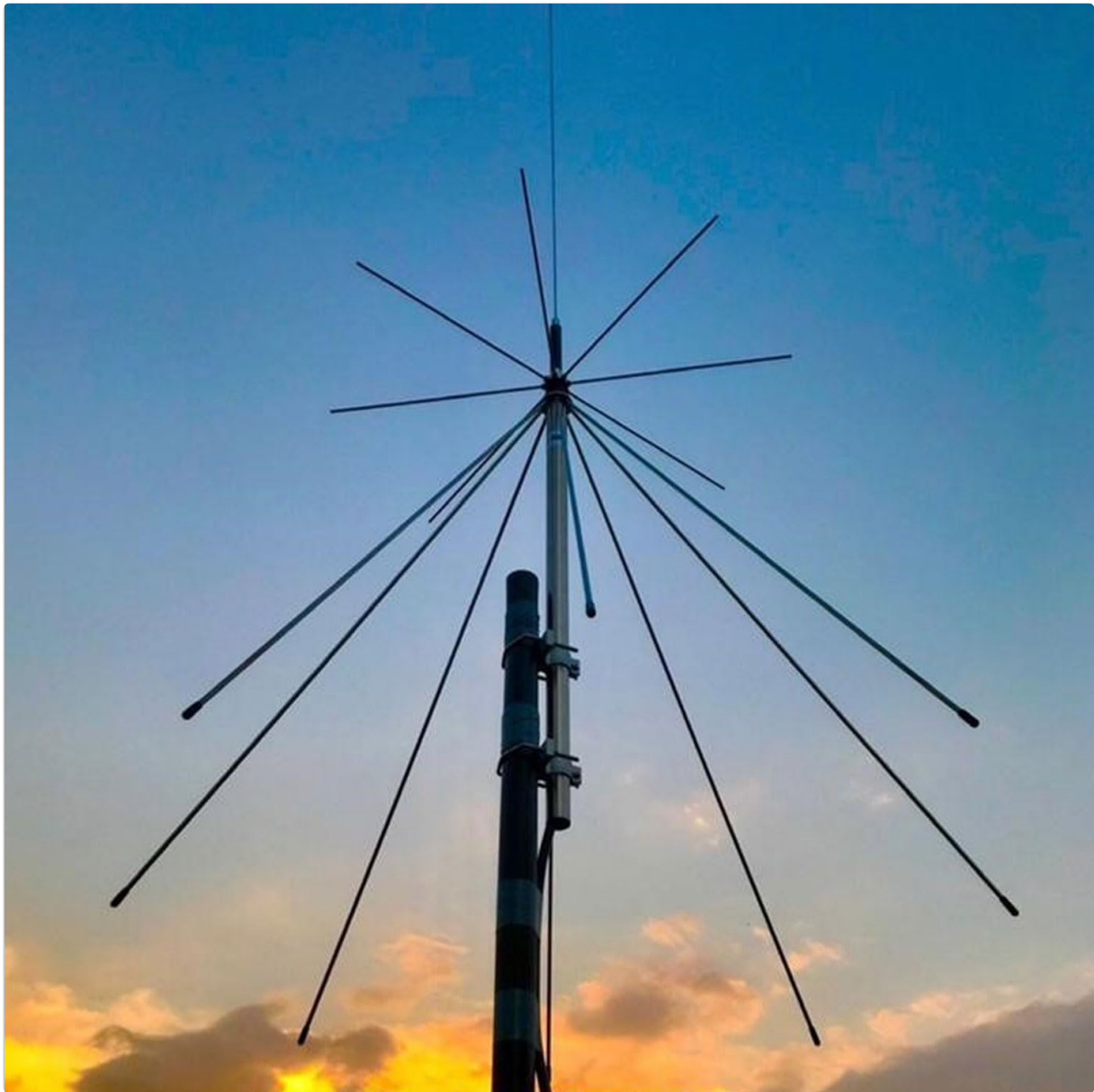
Figure 2.4: The D3000 Discone Antenna mounted on an outdoor pole, illustrating a typical installation scenario.
