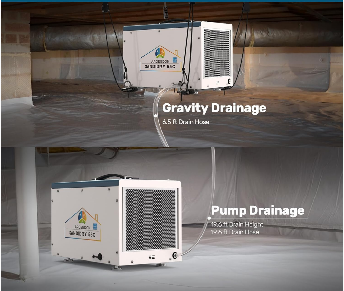
Figure 4.2: Illustration of Gravity Drainage and Pump Drainage setups. The top shows gravity drainage with the unit suspended in a crawlspace, and the bottom shows pump drainage with the unit on the ground.
