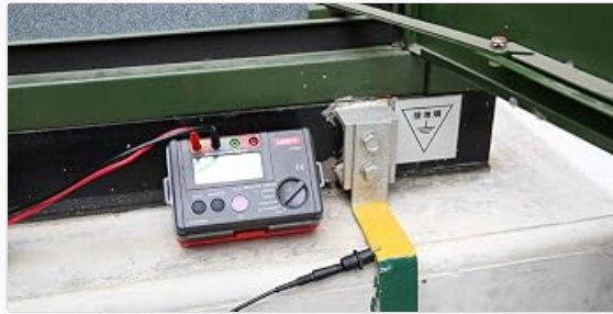
Figure 5: UT526 connected for an RCD test.
