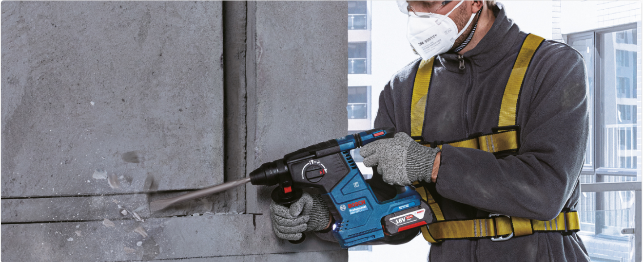
Image: A worker demonstrating safe operation of the Bosch GBH 187-LI, wearing appropriate personal protective equipment including safety glasses and a dust mask, while drilling into a concrete surface.
