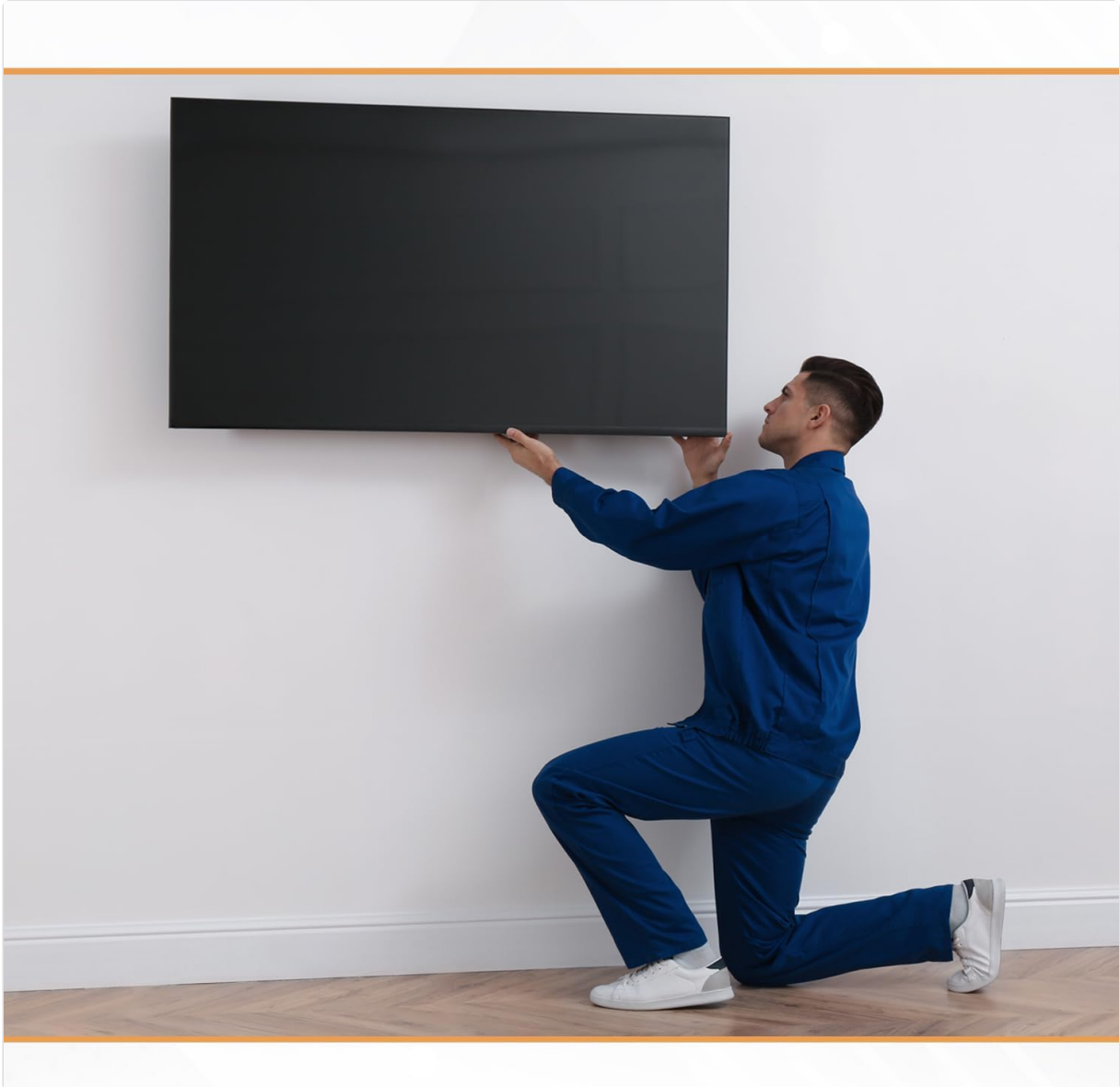
Image: A person carefully lifting a television to attach it to the pre-installed wall mount, illustrating the final step of installation.
