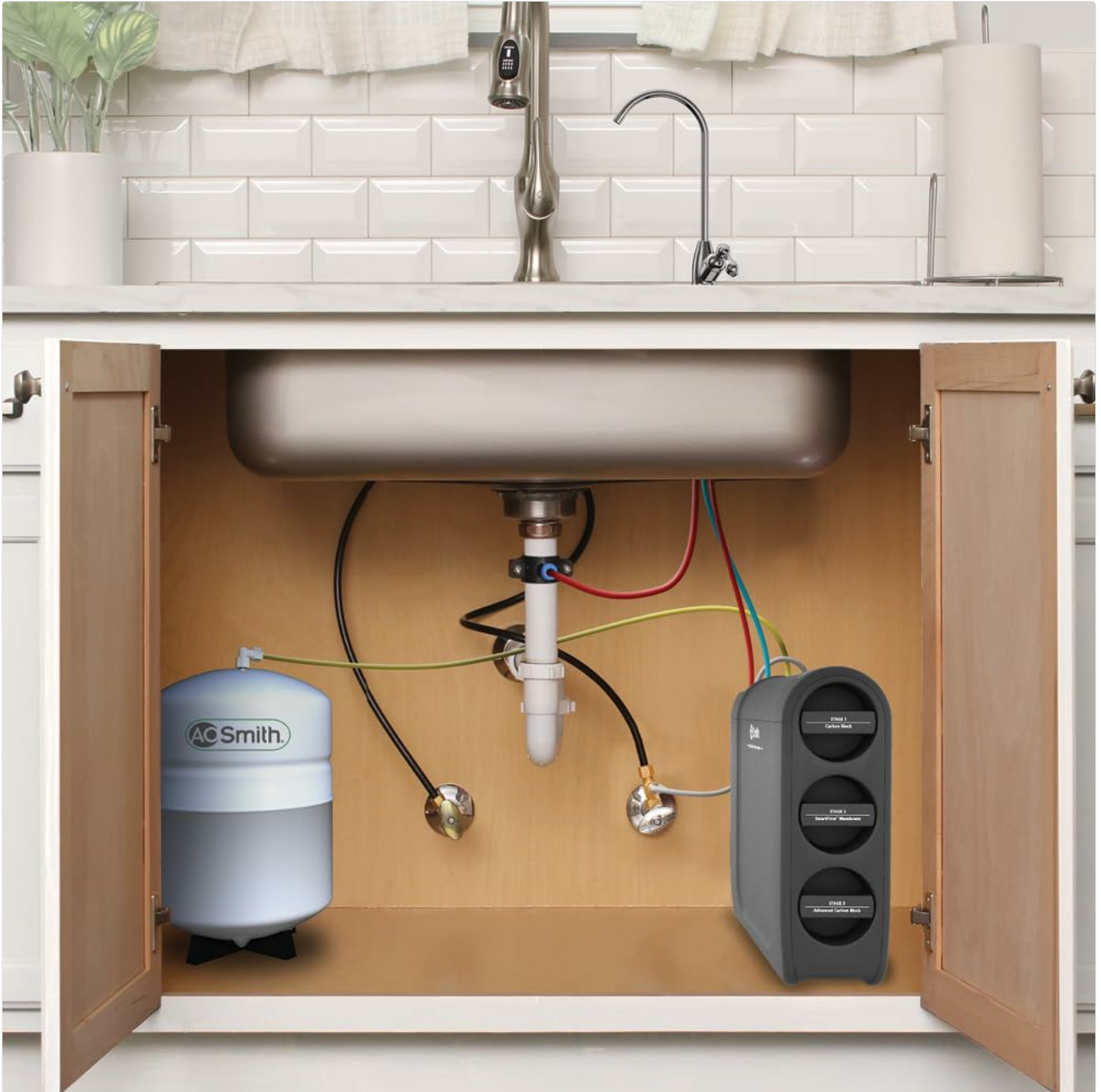
Image: An example of the AO Smith Reverse Osmosis system installed neatly under a kitchen sink, showing the filter unit, the pressure tank, and the connected water lines.
