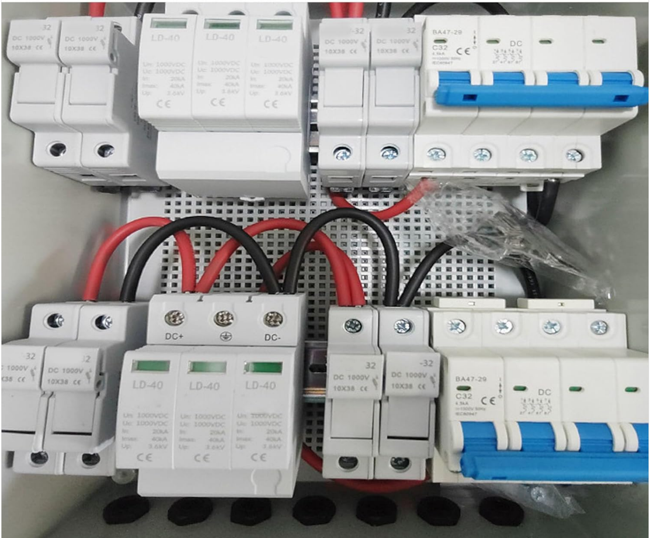
Figure 5: Internal wiring of the combiner box, demonstrating the standard red positive and black negative cable connections to the components.
