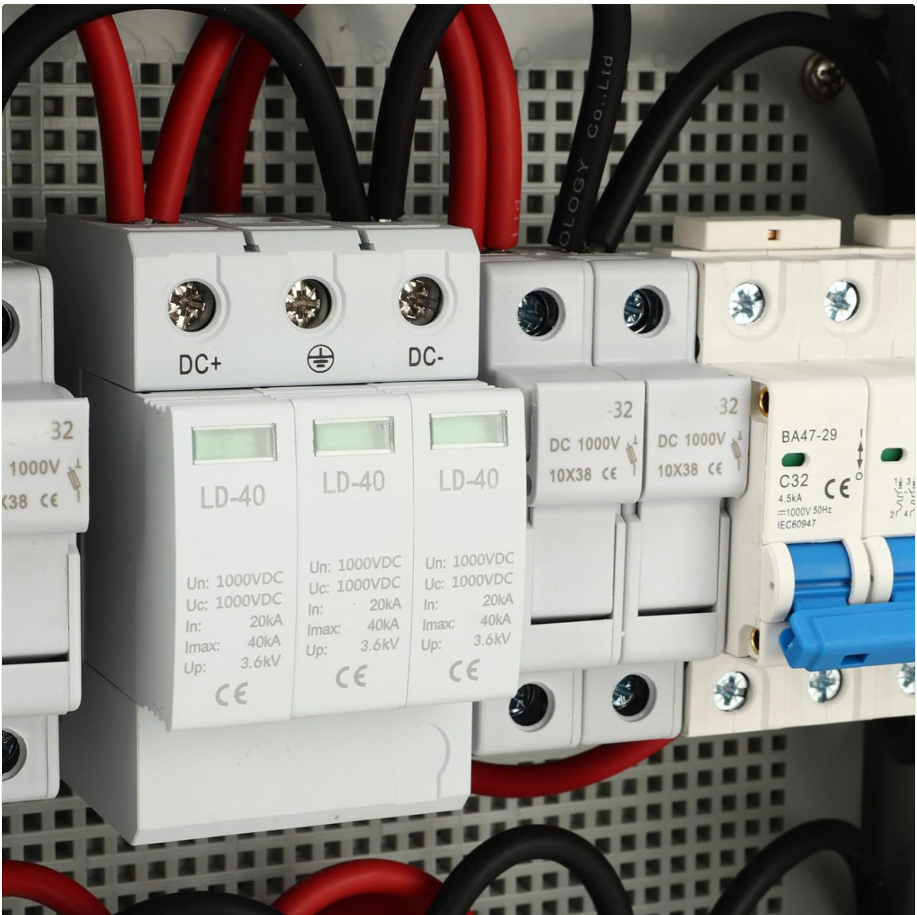
Figure 7: Close-up of the LD-40 surge protective devices, indicating their specifications for DC 1000V, 20kA nominal discharge current, and 40kA maximum discharge current.
