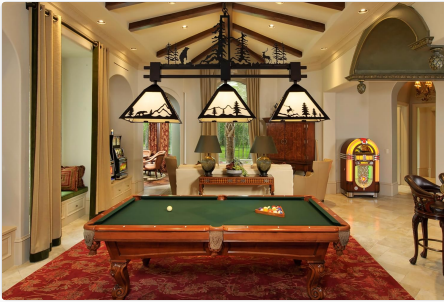
Fixture installed over a pool table.
