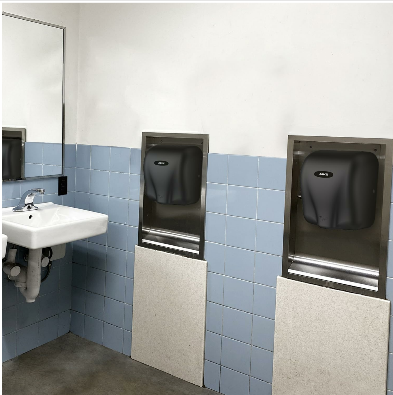
Figure 4: AIKE hand dryers installed in a typical restroom environment, demonstrating placement above sinks.
