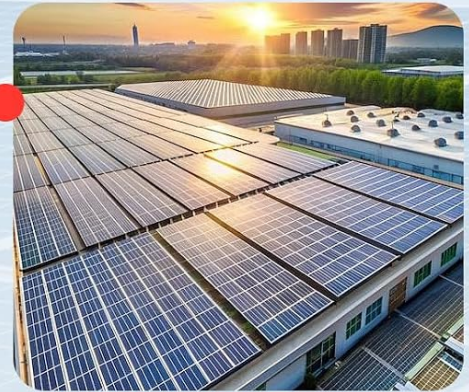
Photovoltaic power station
