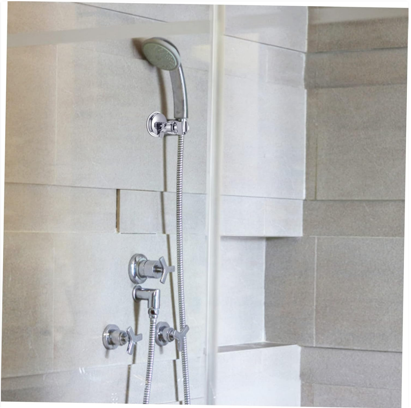
Image: An Alipis shower head holder securely installed on a tiled shower wall, holding a handheld shower head.
