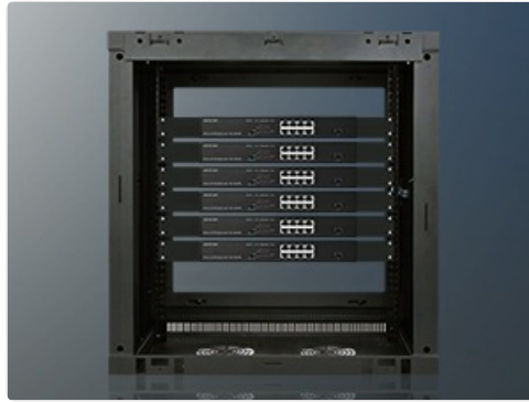
Image: The switch installed in a server rack, demonstrating its rack-mountable design.
