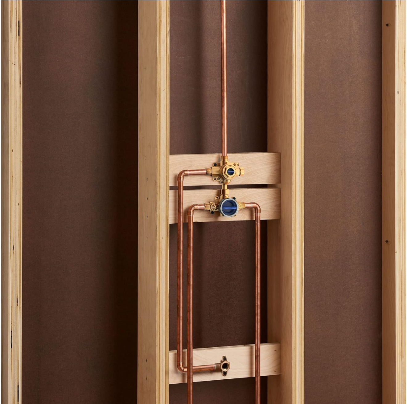
Figure 3: Example of rough-in plumbing with the Grohsafe 3.0 valve installed on a cross brace between wall studs, showing copper pipe connections.
