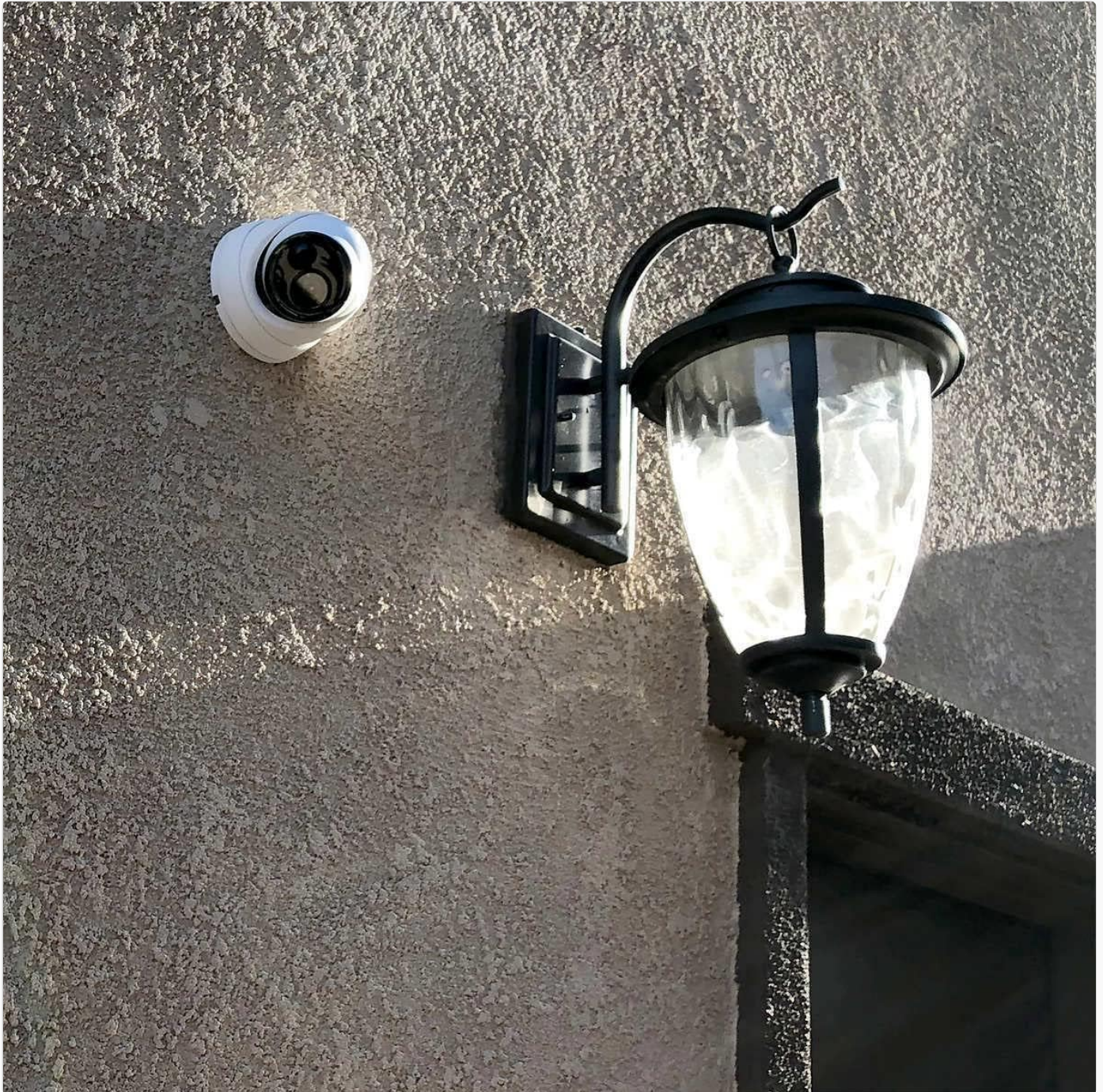
Image: A Swann dome camera mounted on a textured exterior wall, positioned above and to the left of a traditional outdoor lantern-style light fixture.
