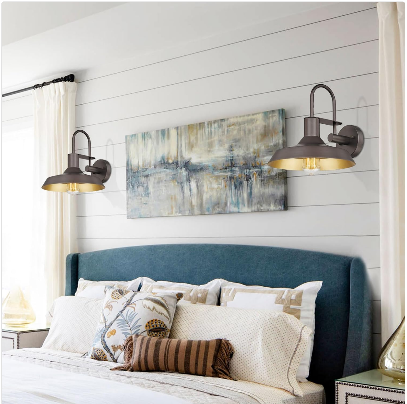
Figure 6: Example of the light fixture installed in a bedroom.
