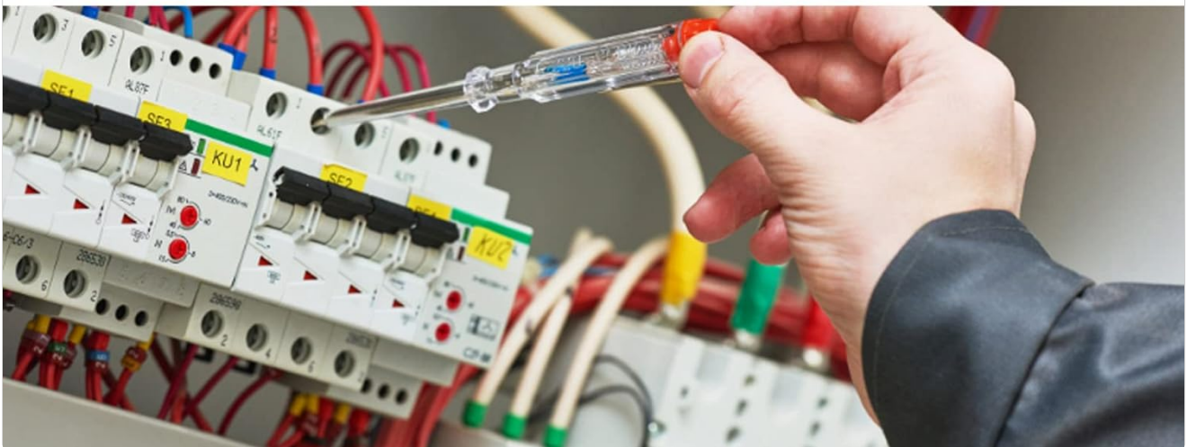
Figure 4: Example of the ATS wired into an electrical panel, demonstrating connections to power sources and load.
