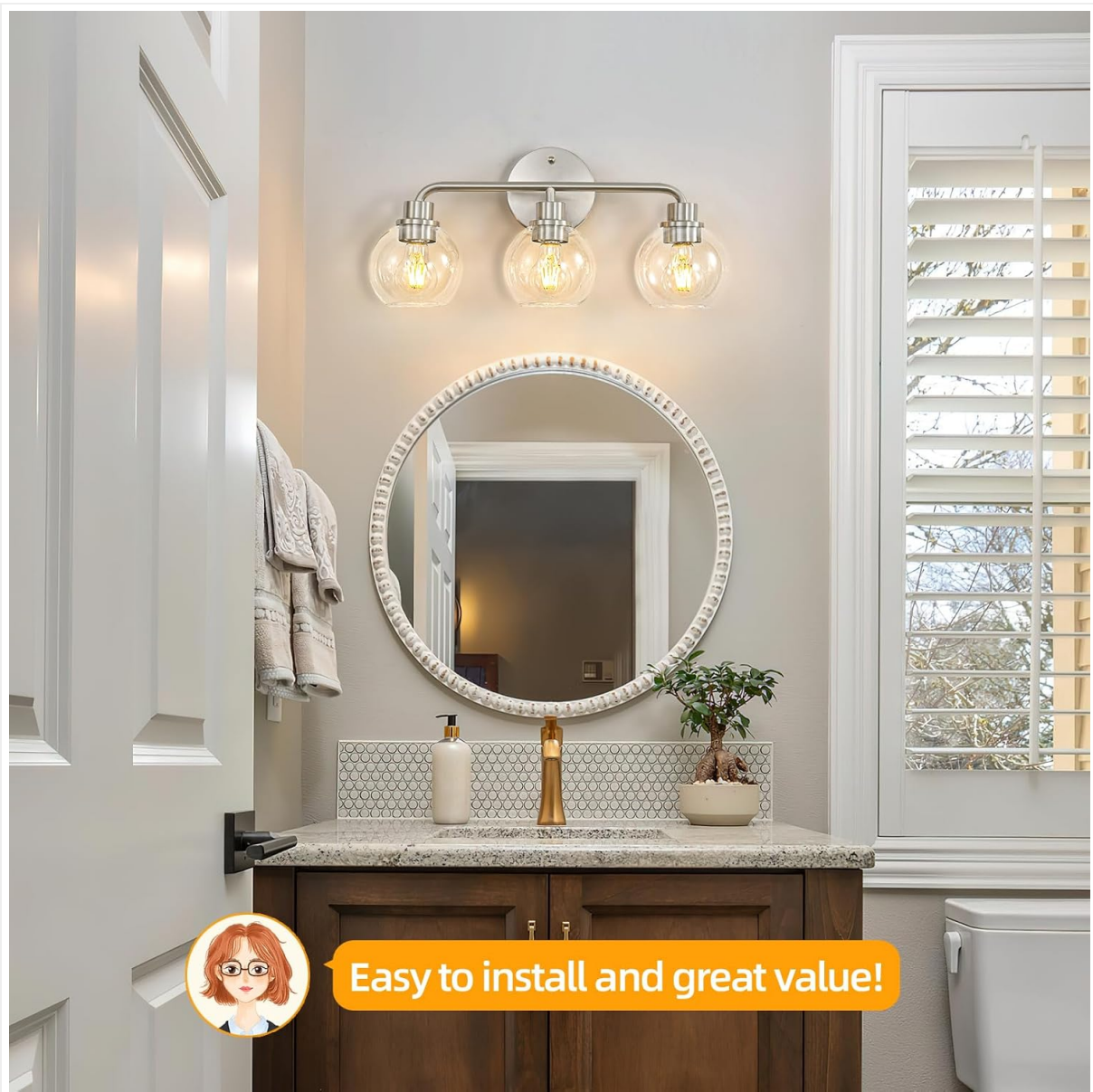
Image: The Watyo 3-Light Brushed Nickel Vanity Light Fixture installed above a bathroom mirror, showcasing its modern design.
