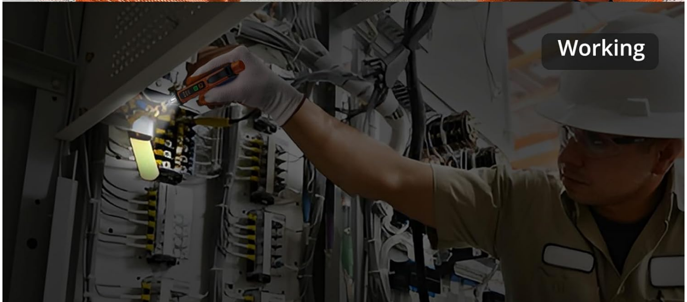
Image 8: The tester's LED flashlight illuminating a dark electrical box, aiding in visibility during testing.
