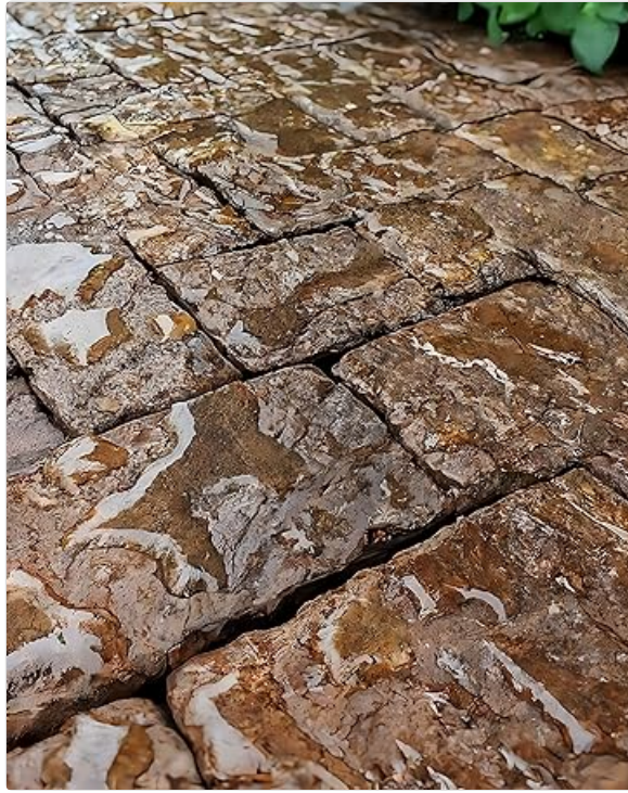
Image 5.3: Coating softening and lifting after CR100 application.
