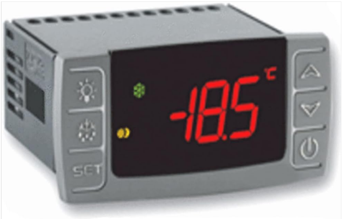
Figure 4: Close-up of the controller's display, showing a typical temperature reading during operation.
