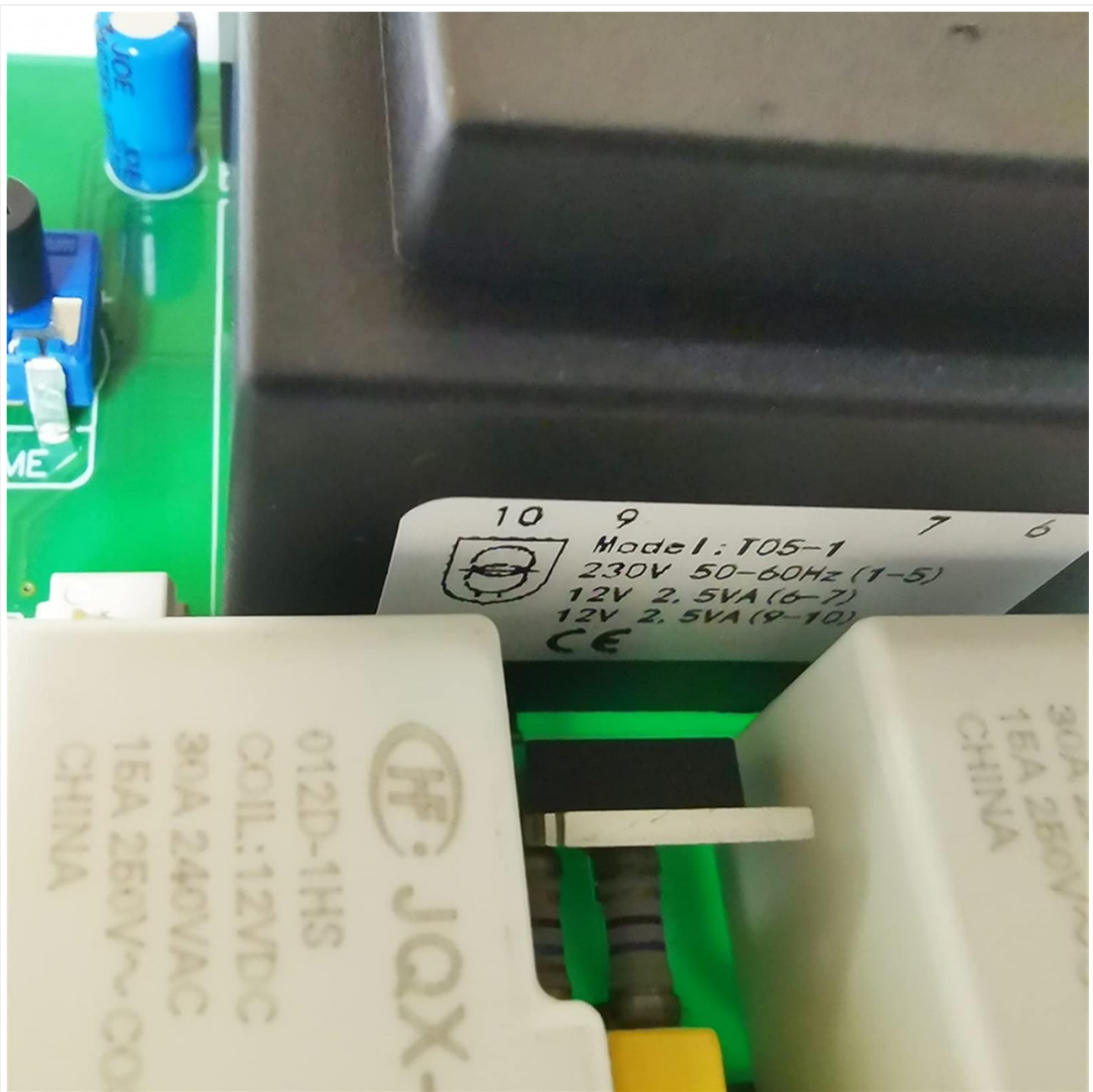
Image 9.1: Close-up view of the transformer label, indicating model and voltage specifications.
