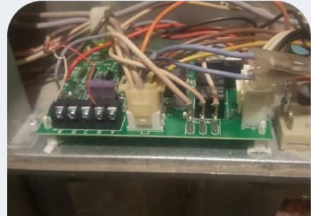
STEP 6 Plugged into new circuit board.
