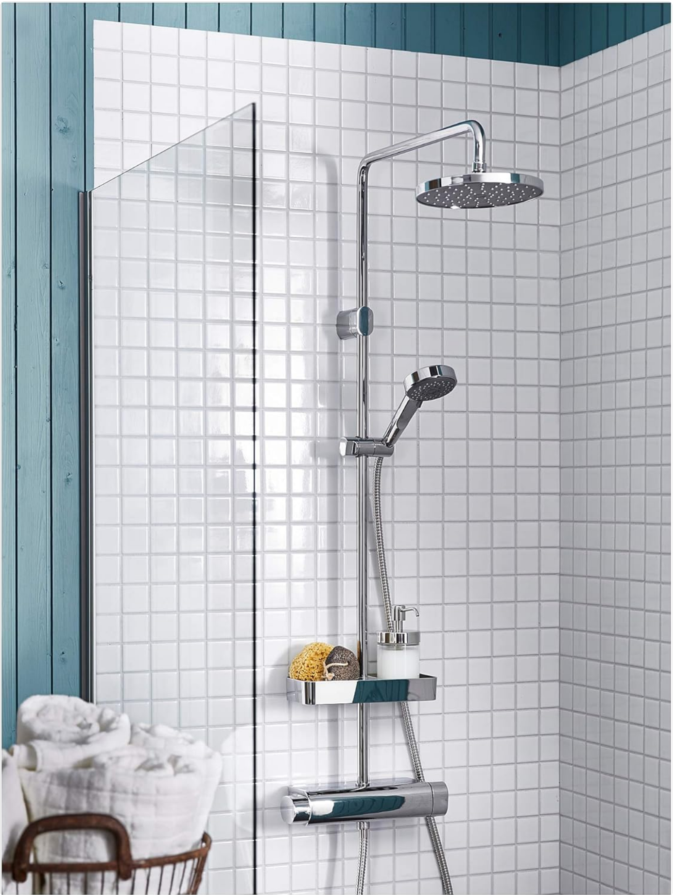
Figure 4: The Ikea Brogrund shower system installed in a modern bathroom with white tiled walls and a blue accent wall. The integrated shelf on the mixer is visible, holding shower accessories.
