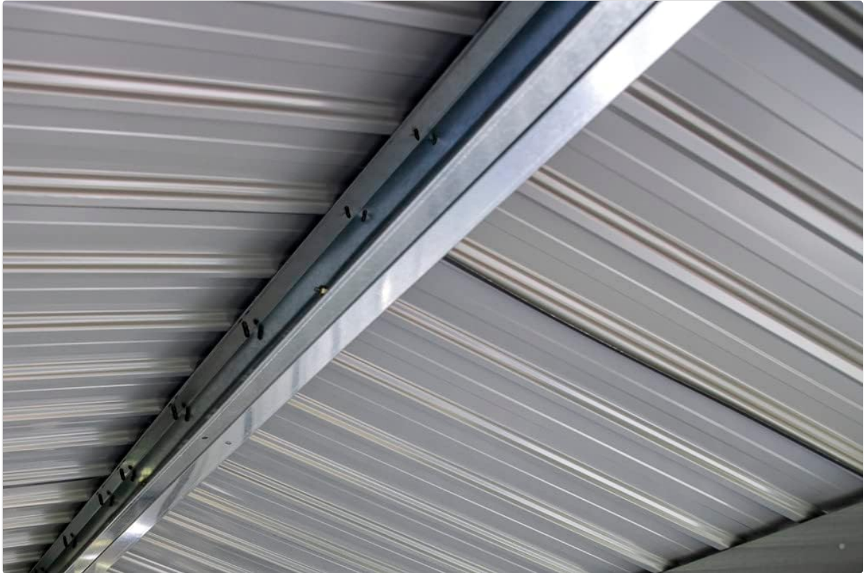
Image 5.1: A detailed view of the shed's gable vents located near the roofline, designed to facilitate air circulation.
