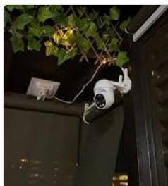
Figure 3: Camera mounted on a building wall.
