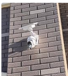
Figure 4: Camera mounted on a brick wall.
