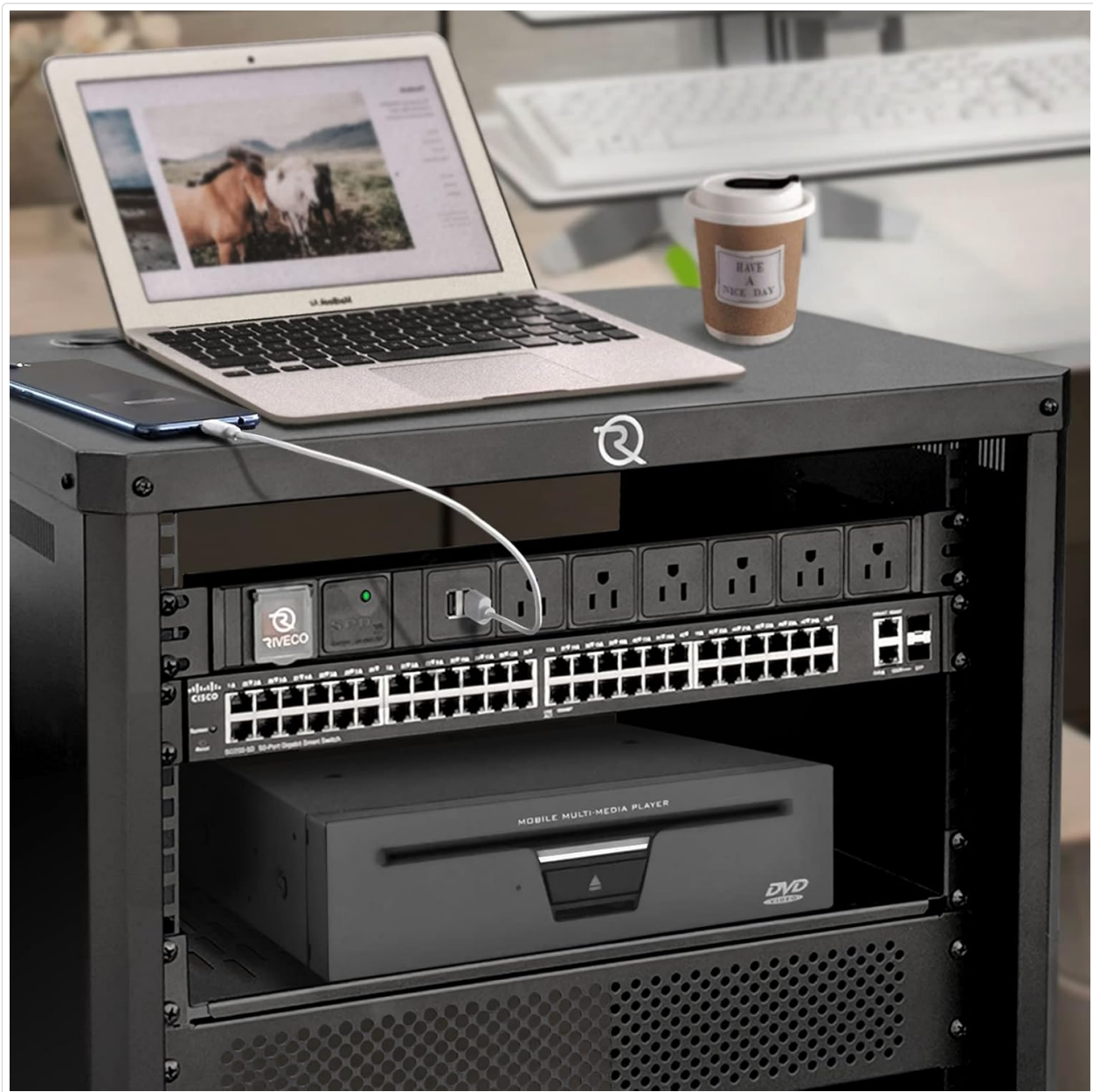
Figure 4.2: An example of the PDU installed in a rack, with a laptop connected to one of the USB charging ports.
